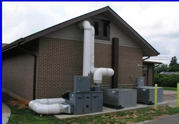
Cold room installed
